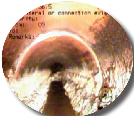
Eventually, as seen above, the grease will begin to close the pipeline all together
