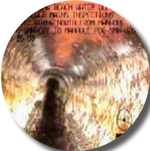
The above photo is an actual photo from the sewer system and shows how grease begins to form inside
